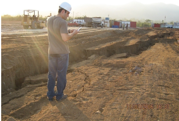
Figure 2.9. Failure of fill with insufficiently long reinforcement
