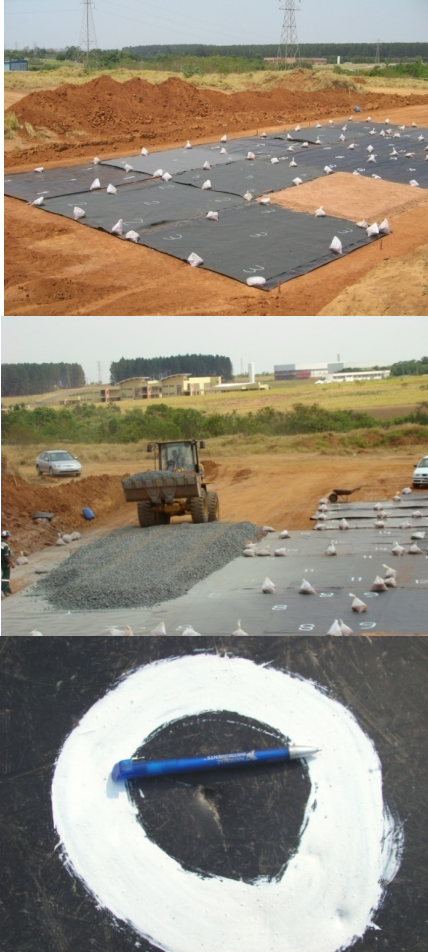
Figure 4.16: Experimental liner construction and example of damage (hole) in exhumed geomembrane (Rebello, 2008).
