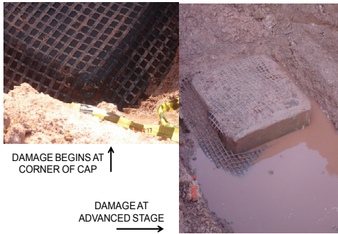
Figure 2.16. Bad behavior of geogrid platform – geogrid torn at cap periphery
