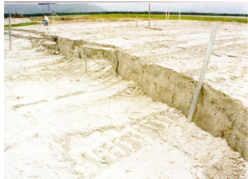
Figure 2.8. Failure of unreinforced fill (Magnani de Oliveira, 2006)
