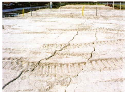
Figure 2.7. Failure of reinforced fill (Magnani de Oliveira, 2006)
