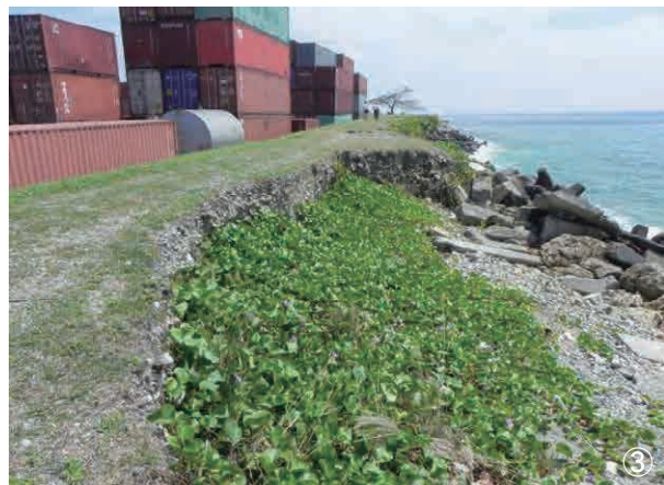
護岸の局所洗掘の状況
