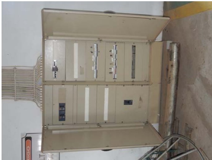
Figure 18. Main Distribution Board, in the Joinery workshop
