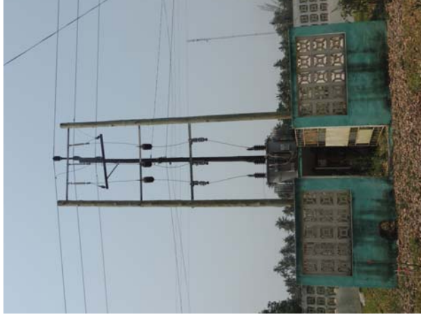
Figure 24. General view of Transformer
