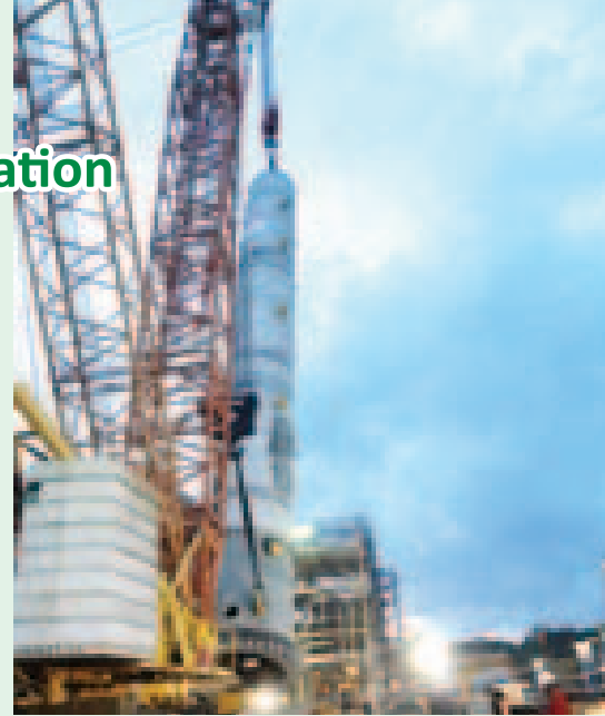
M/s Albanna Engg. The 2nd reactor has also been shifted to site and is scheduled for erection by the end of May 2015.
