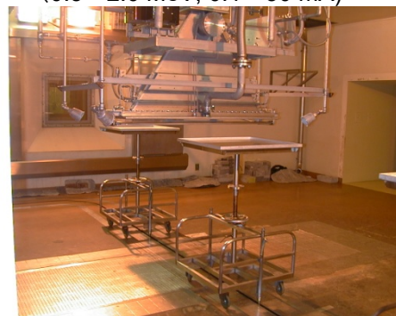
Electron irradiation room with conveyor system
