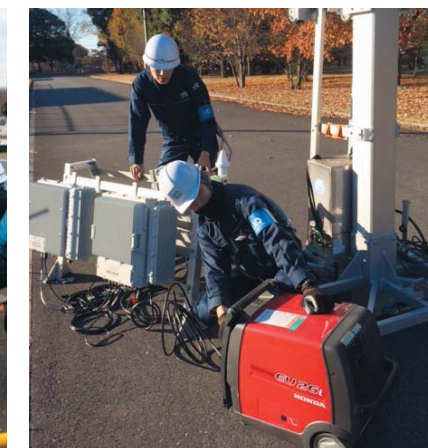
可搬基地局設置訓練の様子 Mobile Base Station Installation and Operation Training
